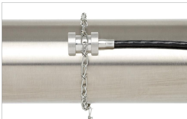
PT100 transducer fixed to pipe
